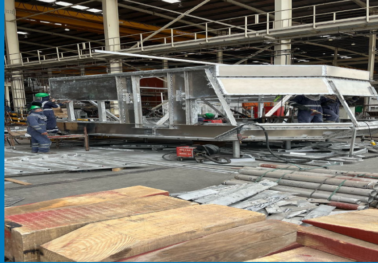
In the picture: Early construction phase of the Wheelhouse for "Kanoo 50", scheduled for delivery in September 2025.
